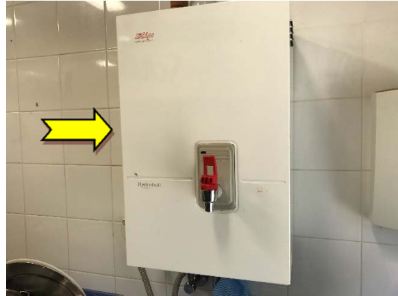
Photo 2. Interior, ground level, kiosk – hot water heater suspected to contain SMF internal insulation.
