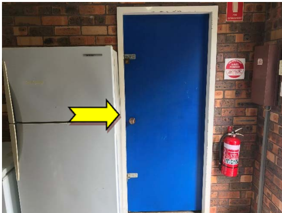
Photo 3. Interior, throughout, doors – suspected lead-containing blue & white paint systems.
