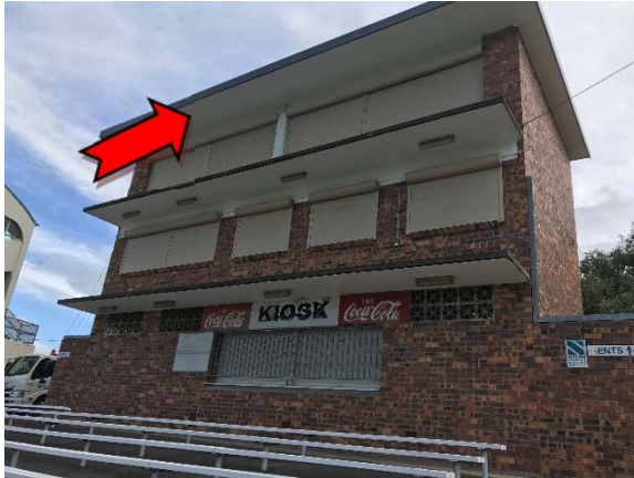
Photo 1. Exterior kiosk, all levels, eaves/awnings – identified/assumed asbestos-containing fibre cement sheeting.
